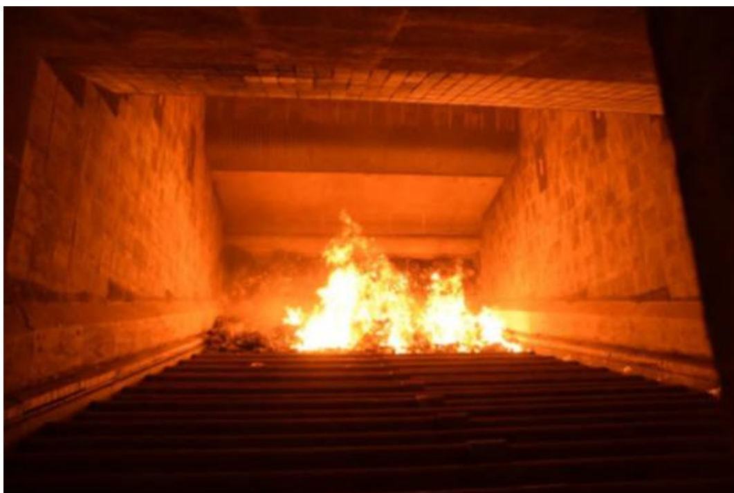
Figure 11: Example of a moving grate combustion system during start-up as waste is being fed onto the moving grate
